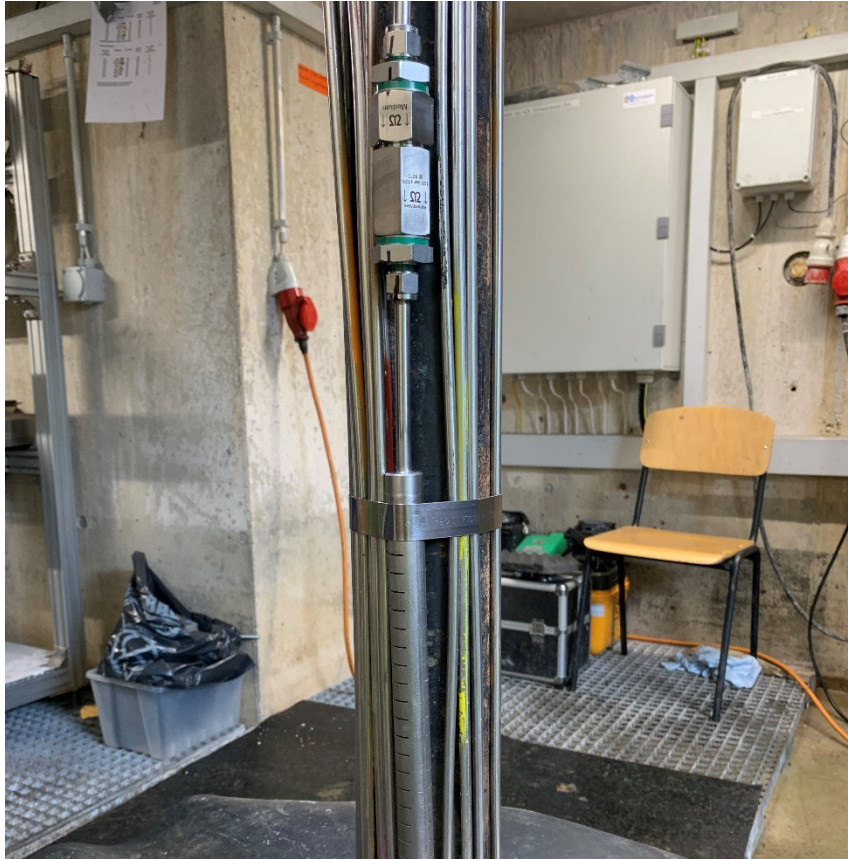
Fig. 2-4: Filter port with burst disc above, installed on the central tubing with metal banding straps
