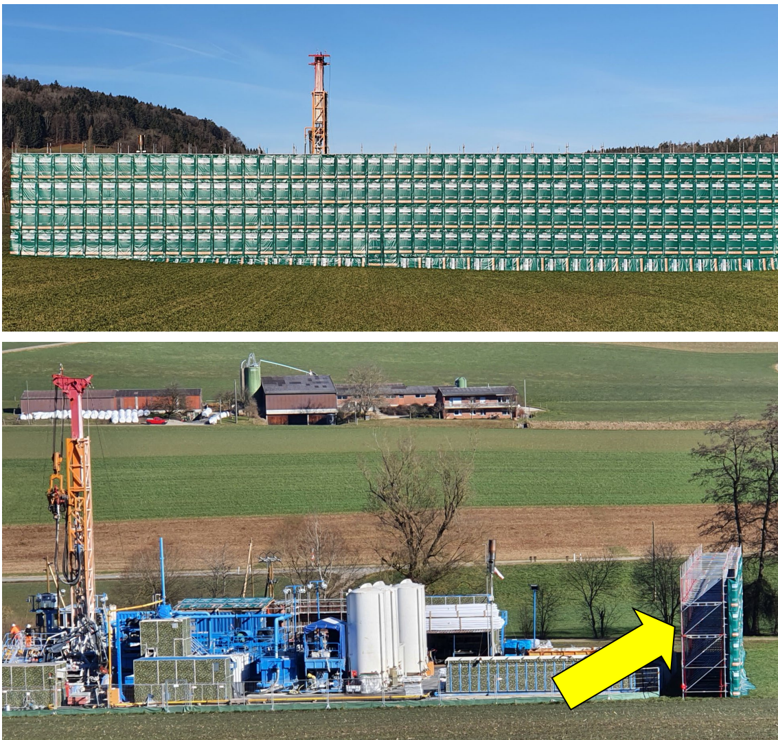
Fig. 3-21: Noise protection wall at the south-eastern side of the drill site
