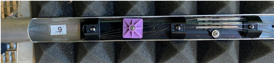
Fig. 2-7: View of the opened splice box with three splices of the FO cable
